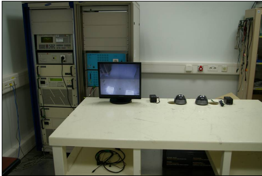
Picture 5. Harmonics & Flicker
